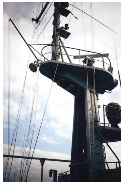
FIG 2 Antenna system of maritime radio station Photos: Force Navale
